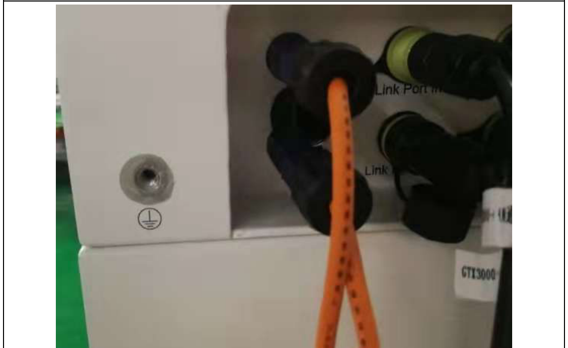
General view of Grounding terminal
