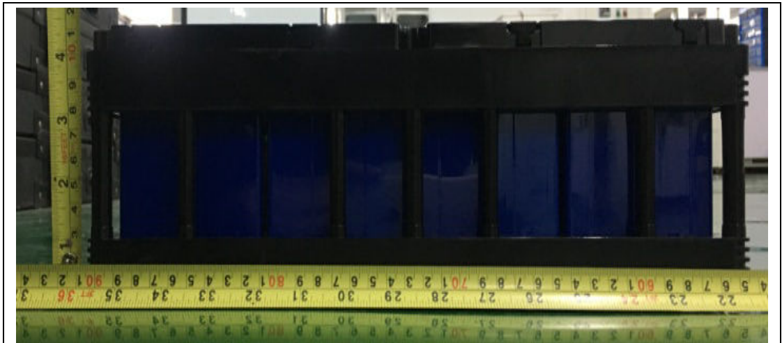
Battery cells general viwe -2 of battery expansion modules
