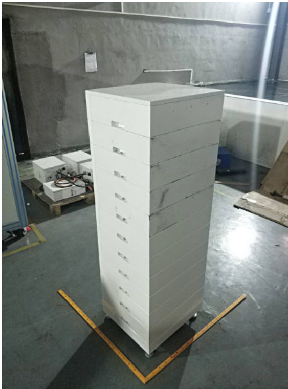
General view-2 of battery
